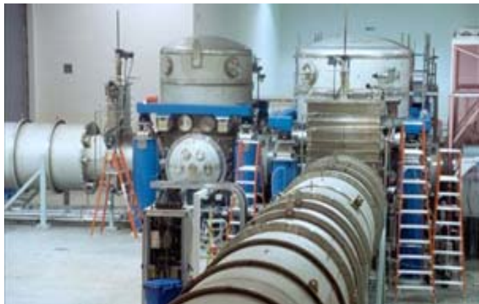
A view of the high-vacuum vertex chambers at the Livingston, LA site (bottom). Credit: LIGO Laboratory.
