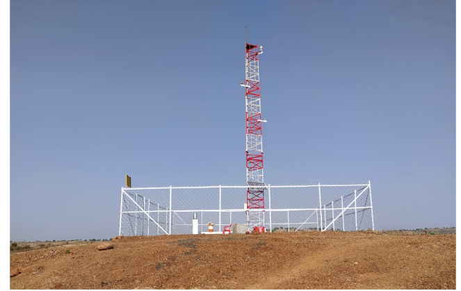
Weather station at the LAO site
