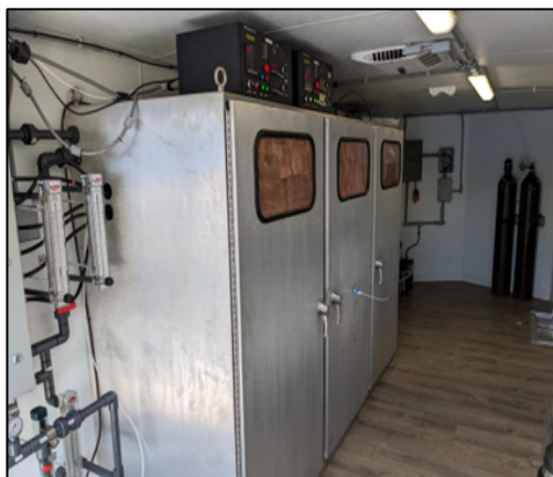
Large volume perfluorinated substance (PFAS) treatment
