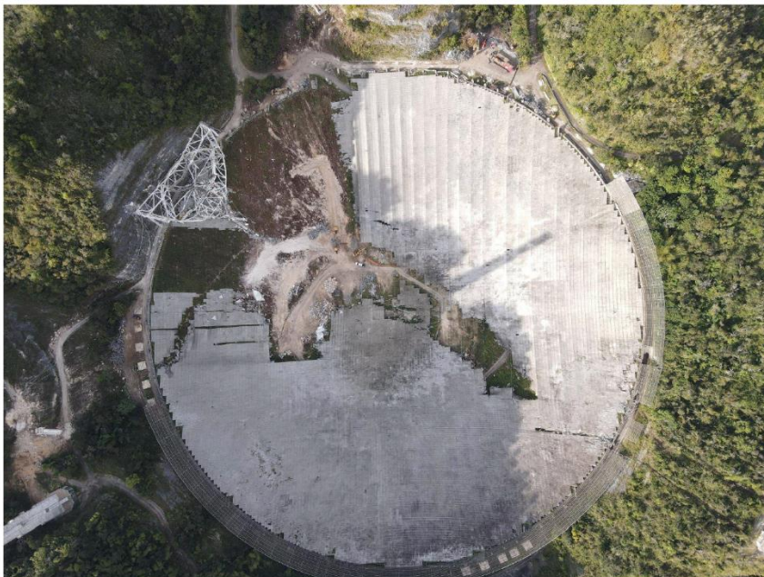
Figure 2: An overhead image illustrating the portions of the reflector and support structure damaged by the collapse. This photo was taken after the cleanup process was well underway so much of the debris
