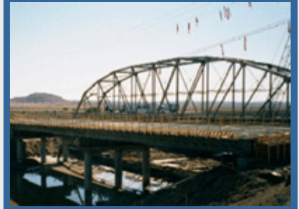
The Rio Puerco bridge outside of Albuquerque, New Mexico, was built with embedded fiber optic sensors to monitor vibration and wear.
